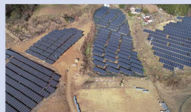
Okayama Prefecture Takahashi No.2 Power Station
